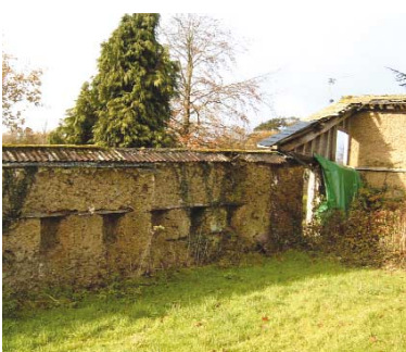
many pigeon holes pockmark the back courtyard.
